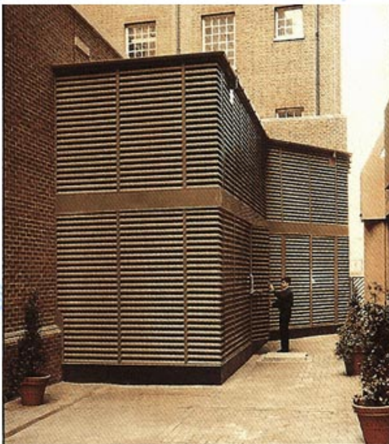
WLAC100 steel louvres around a diesel generator
